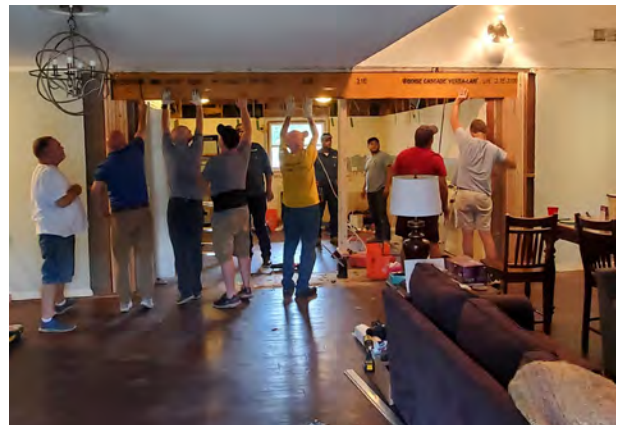
Volunteers from Clearview Baptist Church pitched in to complete a much-needed kitchen remodel in one of our Brentwood homes.
